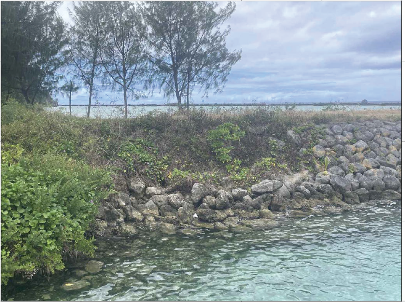
Figure 4. Photo of revetted mole damage in need of structural repair at Station 0+00 to 0+50. Photo taken from harbor side facing ocean side.
