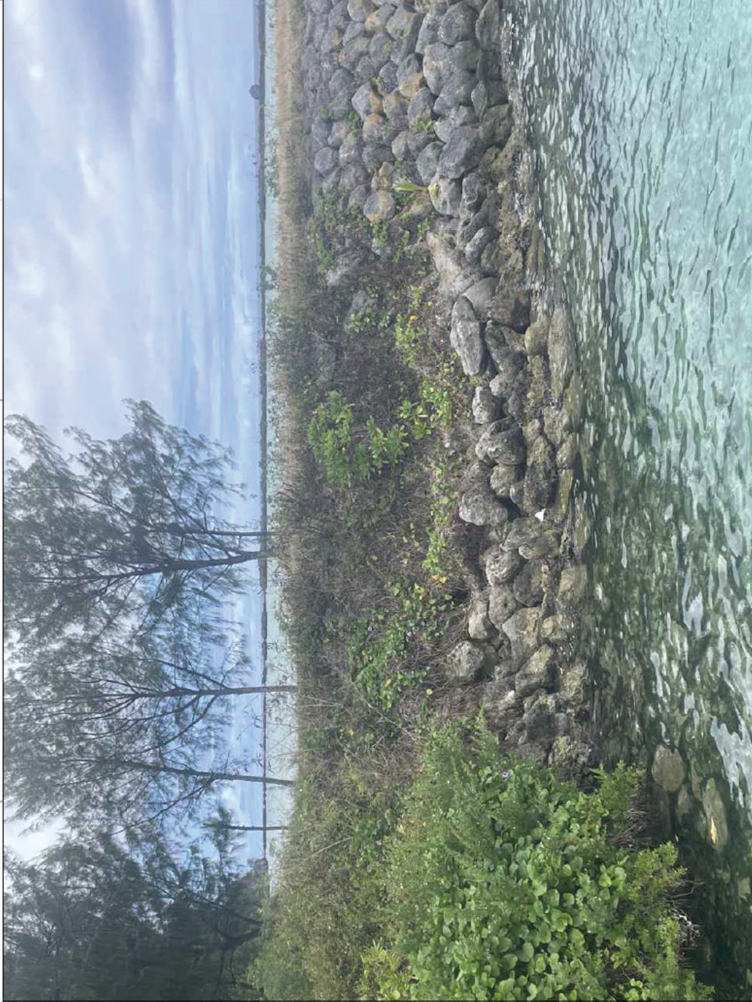
Figure 4. Photo of revetted mole damage in need of structural repair at Station 0+00 to 0+50. Photo taken from harbor side facing ocean side.
