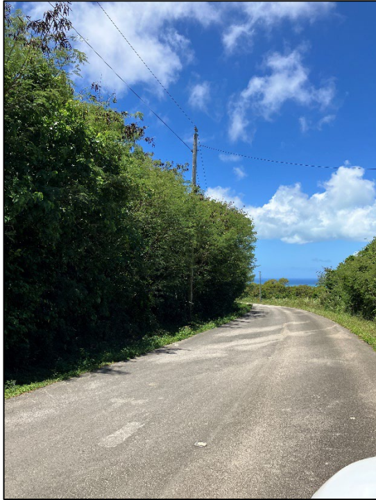
Picture 5: Existing single-phase electrical line distribution (ELD) wooden poles along Pale Arnold Road.
