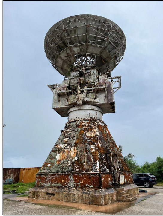
Picture 30: PACBAR III Radar Array
