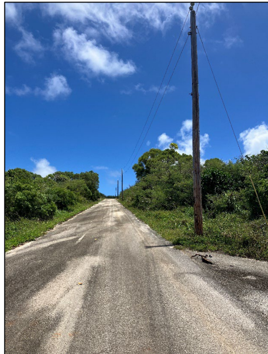
Picture 4: Existing single-phase electrical line distribution (ELD) wooden poles along Pale Arnold Road d.
